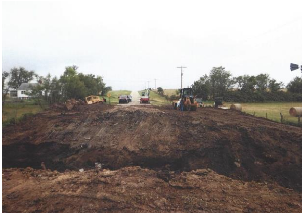
Flash flooding washed out a drain tube on the PBPB Reservation main arterial road. Photo taken on June 4, 2015, by PBPB Road and Bridge staff.
