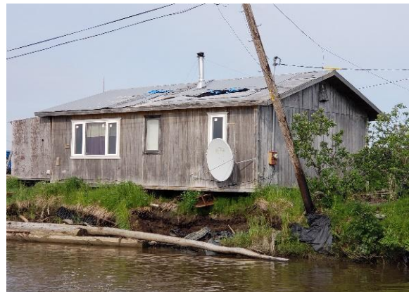
Home affected by permafrost and erosion and that is a first priority to move away from the riverbank. However, it cannot be moved due to an unstable foundation.
